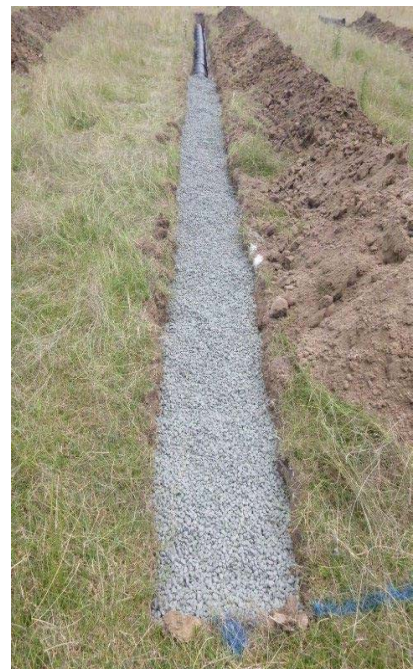
An example of good OSSM practice. A Reln trench connected to a septic system. The trench is in a long straight line with a 100mm layer of blue metal allowing for greater absorbancy and volume capacity.
