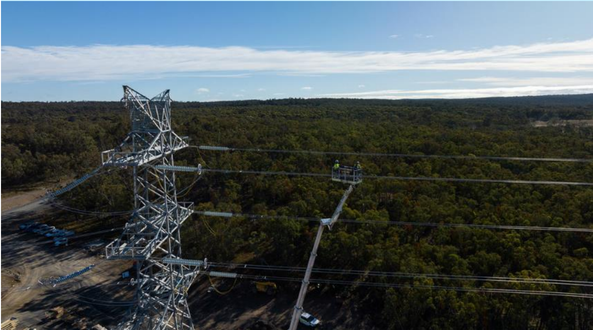
(Image Source: Powerlink)
