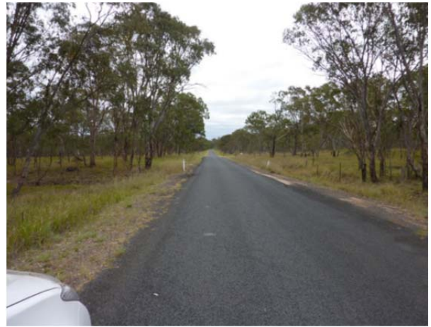
Sealed Road – Condition 2 (Torryburn Road)
