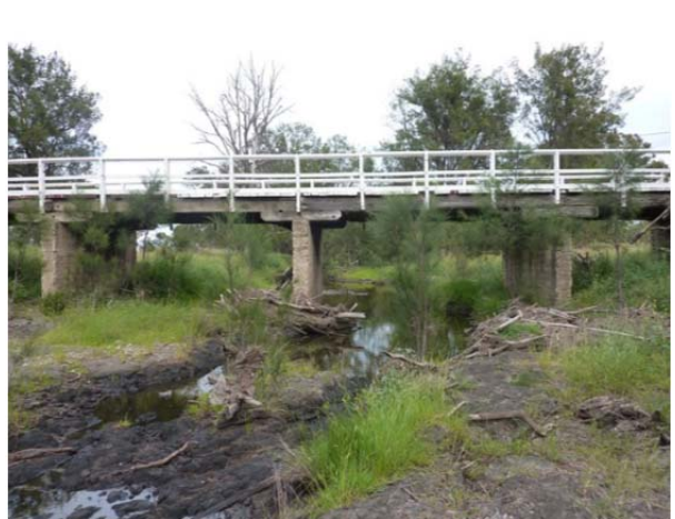
Timber Bridge due for replacement
